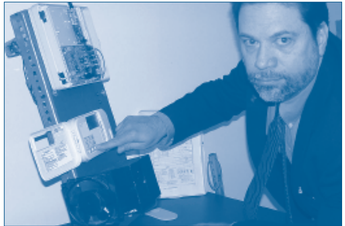
Energy Manager Ron Balon with a test unit for HVAC controls.
