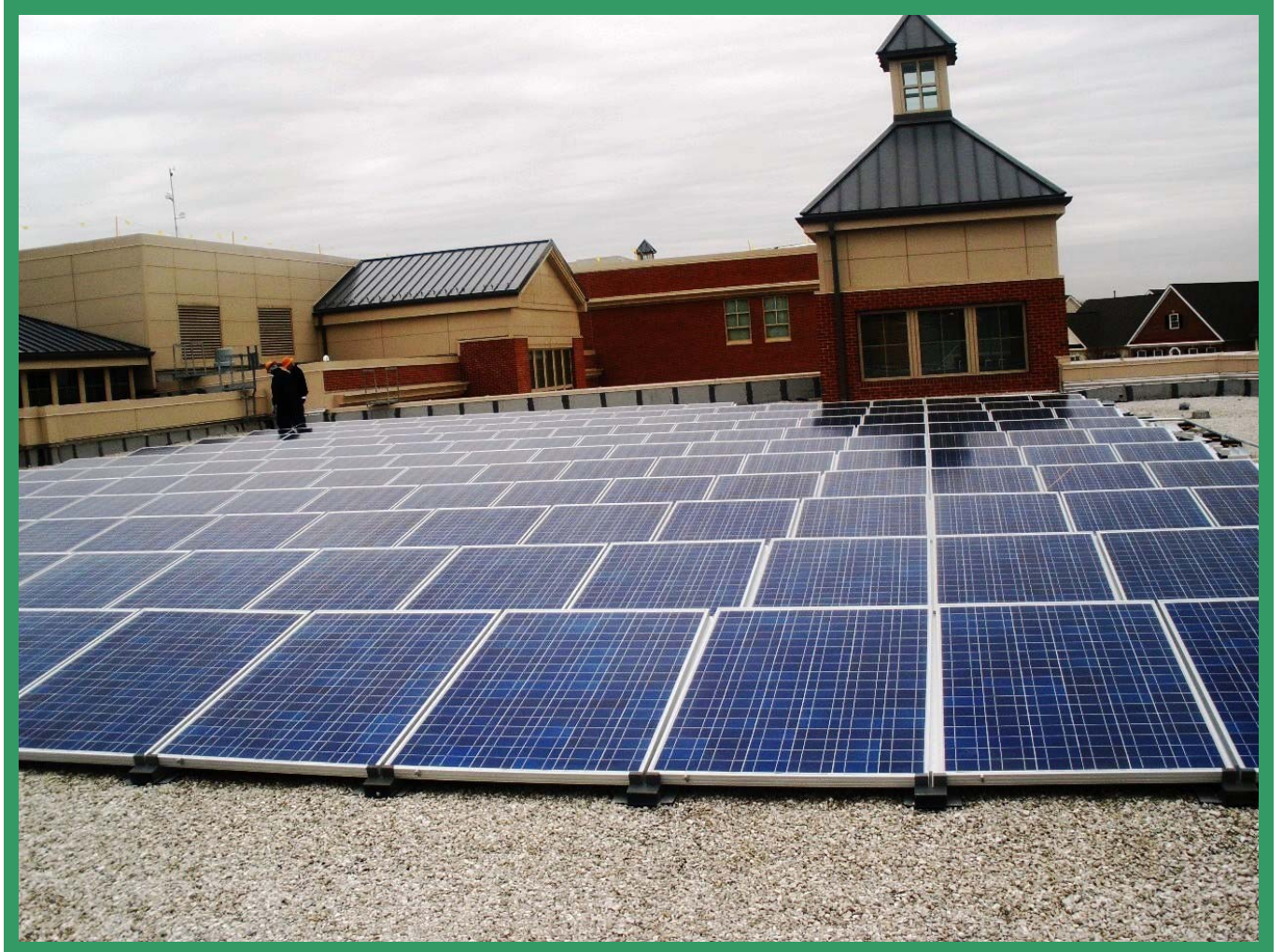
Pictured above: Section of Lakelands Park Middle School Roof Part of 133 kW Solar Photovoltaic System Installed by Power Purchase Agreement in 2008
